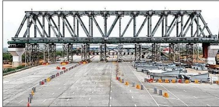
The steel bridge has been launched near the under-construction toll of the Delhi-Mumbai National Expressway near city
